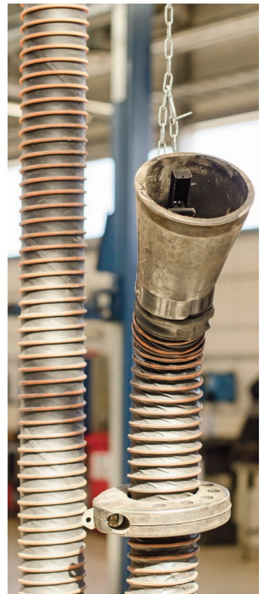
Adjustable and mobile local exhaust ventilation for exhaust pipes in a workshop where vehicles are tested in operation.
